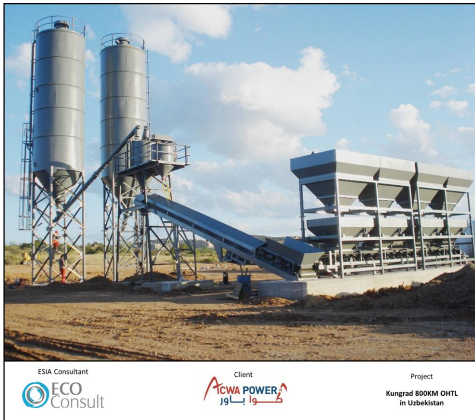
Figure 15: Typical Mobile Batching Plant
