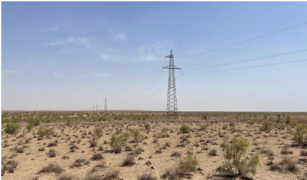
Plate 14-2 Existing Overhead Transmission Lines
