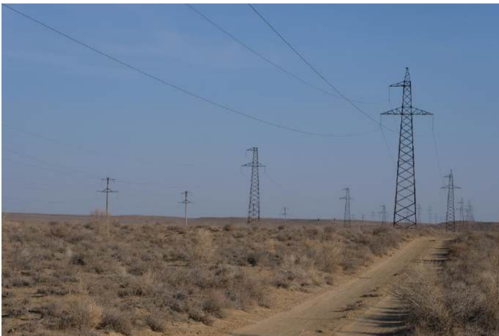
Plate 12-3 OHTLs in the Project Site
