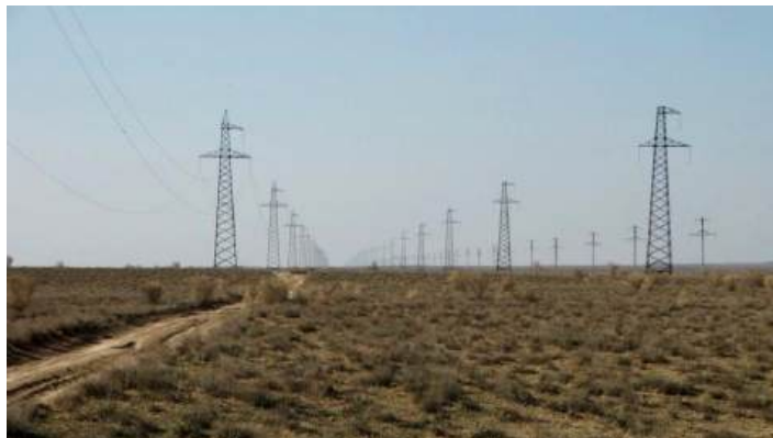
Plate 2-6 Overhead Transmission Lines at the Project site
